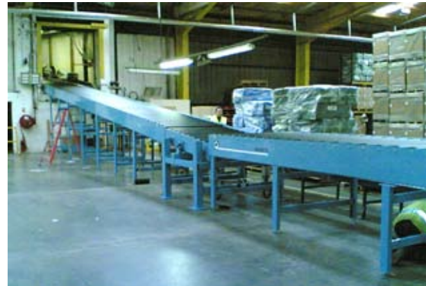
View of conveyors exiting link and into warehouse.
